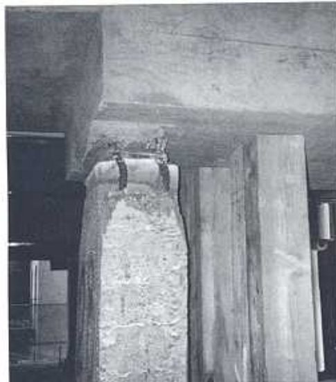
Photo 1: Column damage included buckled reinforcing bars.
